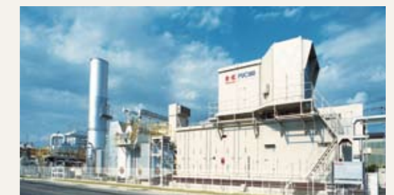
Gas turbine generation system at Akashi Works
